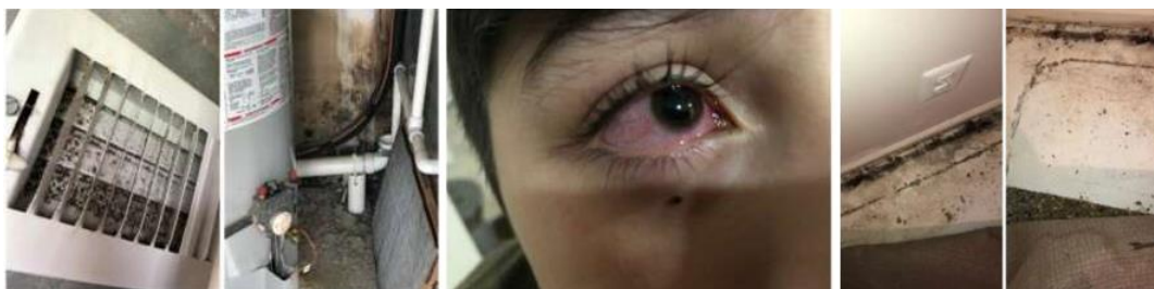
HVAC closet and vent (left) covered in mold in Ft. Meade housing, child's irritated eyes, and (right) other mold areas (photos from lawsuit documents)
